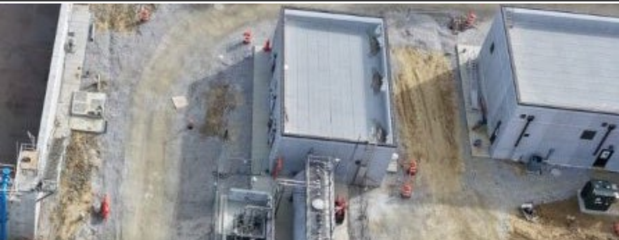
Fully commissioned Methanol facility
